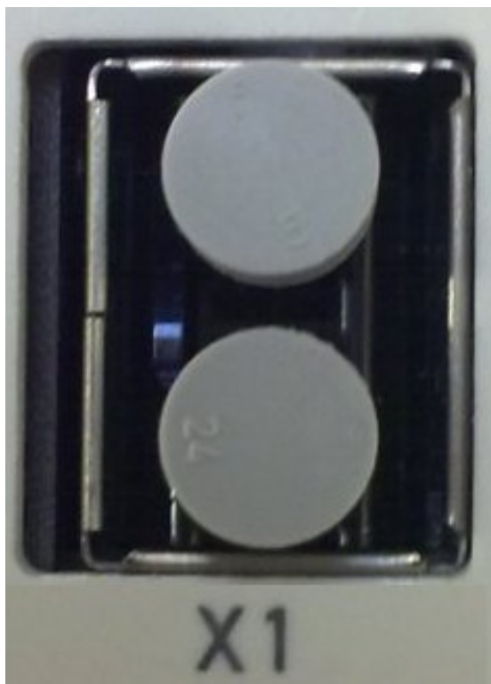
Fig. 32: Blind plugs in unused sockets
